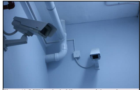
Figure 43 CCTV at the holding area of the station
