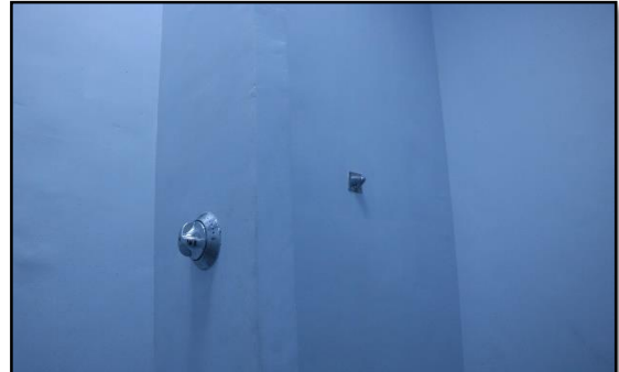
Figure 41 Shower facilities provided for the detainees
