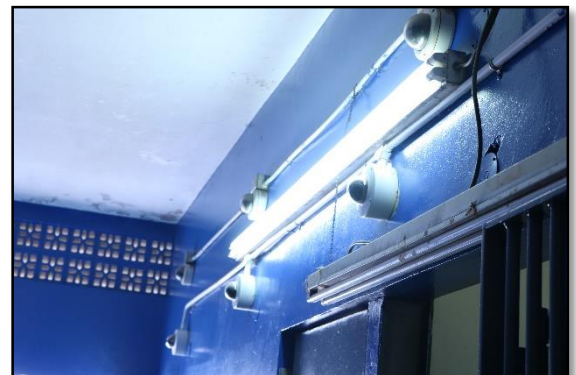
Figure 22 Positioning of the lights and cameras at holding cell area of the Chaguanas Police Station
